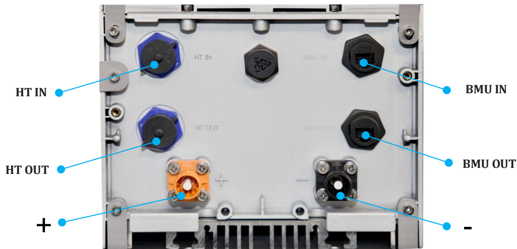
Figure 5.34 Battery Module Wiring Panel
